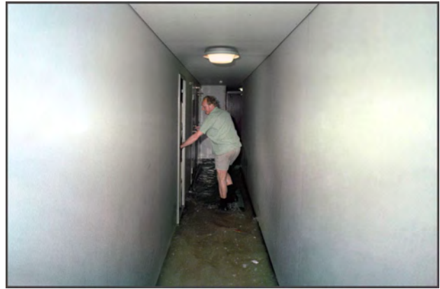
"Stolt Surf" — water filled alleyways — Chief Steward Erik Schønnemann inspecting the crew's accommodation for damage (Photography by Karsten Petersen ©)
